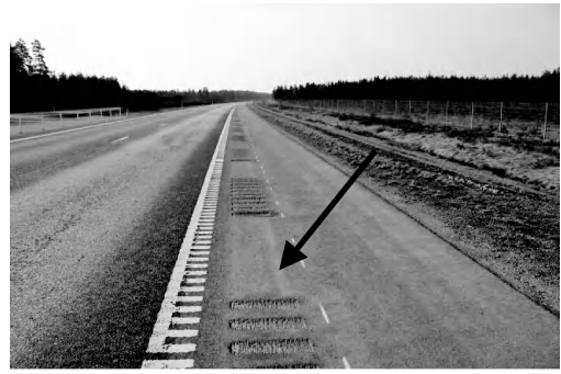
Figure 8.3 Rumble strip milled into the road surface at the shoulder. (See color plate section).
